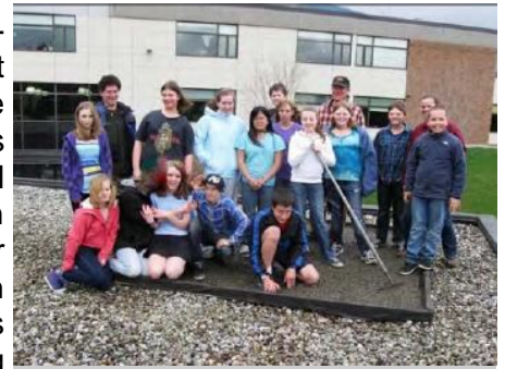
U-32 students pose for a picture with their freshly installed nest patch.
